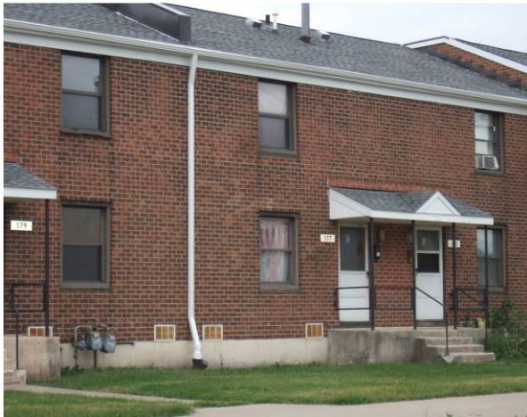
One of the row houses of the Perry Projects near the Buffalo Creek Casino
