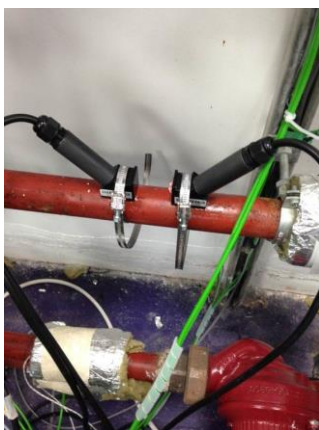
Figure 4 Image showing the installation method of transducers
