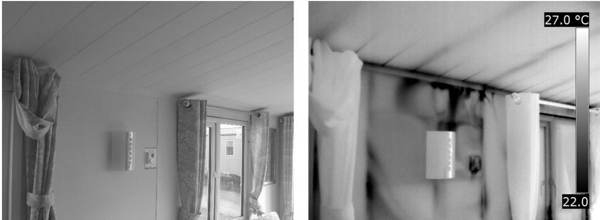
Figure 8 Indirect air leakage around electrical cable runs.
