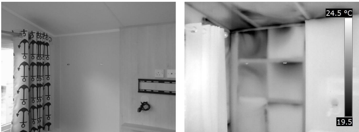
Figure 9 Indirect air leakage through external wall.
