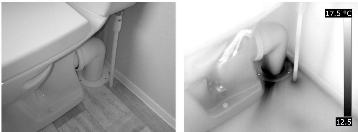
Figure 4 Direct air leakage around the toilet waste pipe
