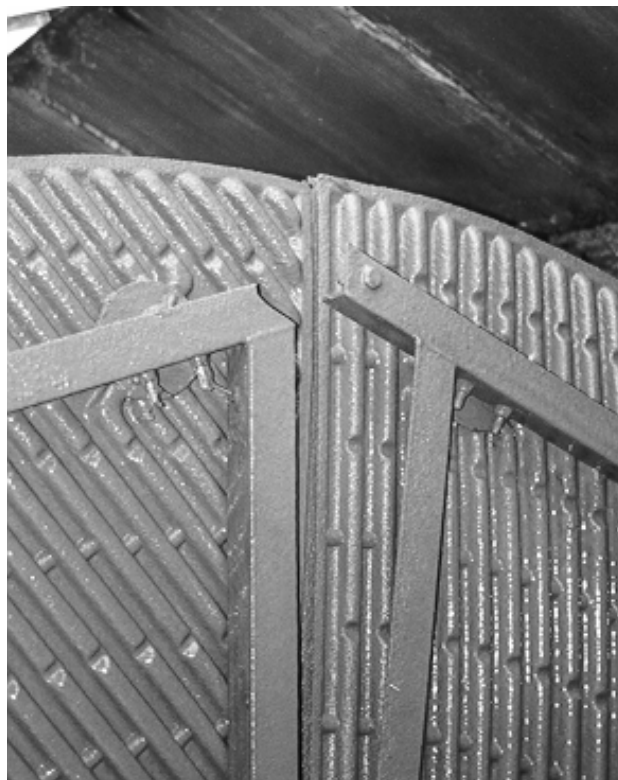
Figure 59 Fractured support structure
