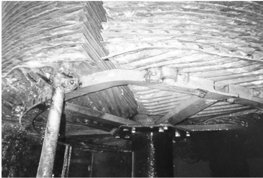
Figure 67 Bend support structure
