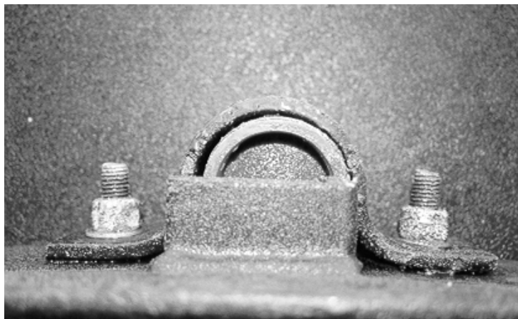
Figure 68 Inadequate clamping of through rods plus axial end stop
