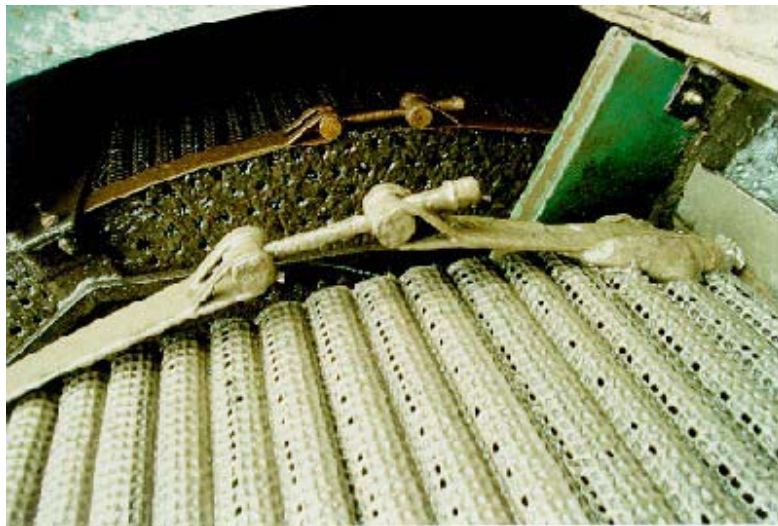
Figure 38 Loose outer circumferential strap
