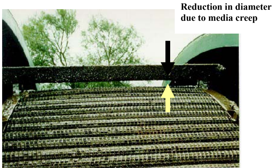
Figure 39 Gap between structure and media coils caused by media creep
