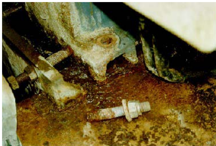
Figure 40 Fracture of foundation bolts due to transient torque produced by loose media pack
