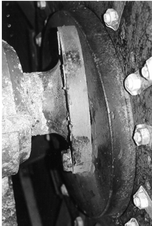
Figure 102 Complete collapse of RBC unit due to fracture of stub shaft coupling bolts
