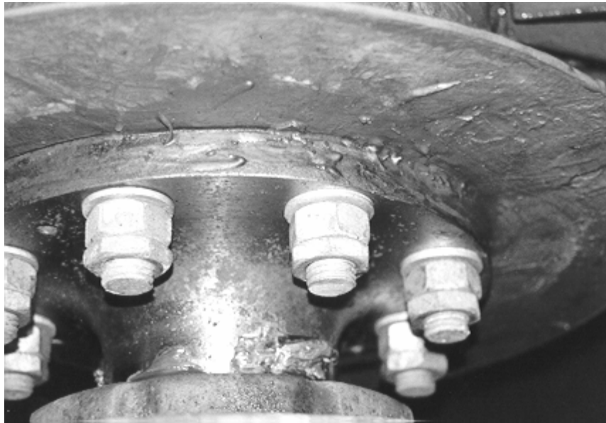
Figure 76 Improper bolting of double lock nuts
