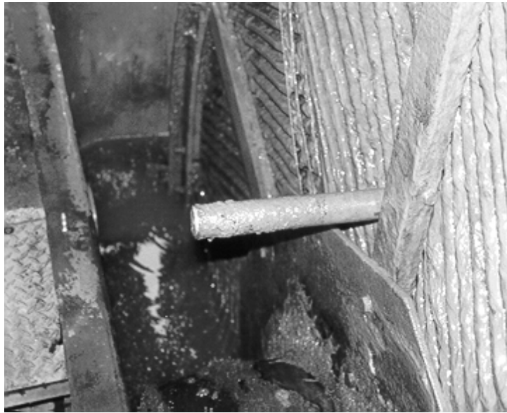
Figure 63 Loose inner through rod
