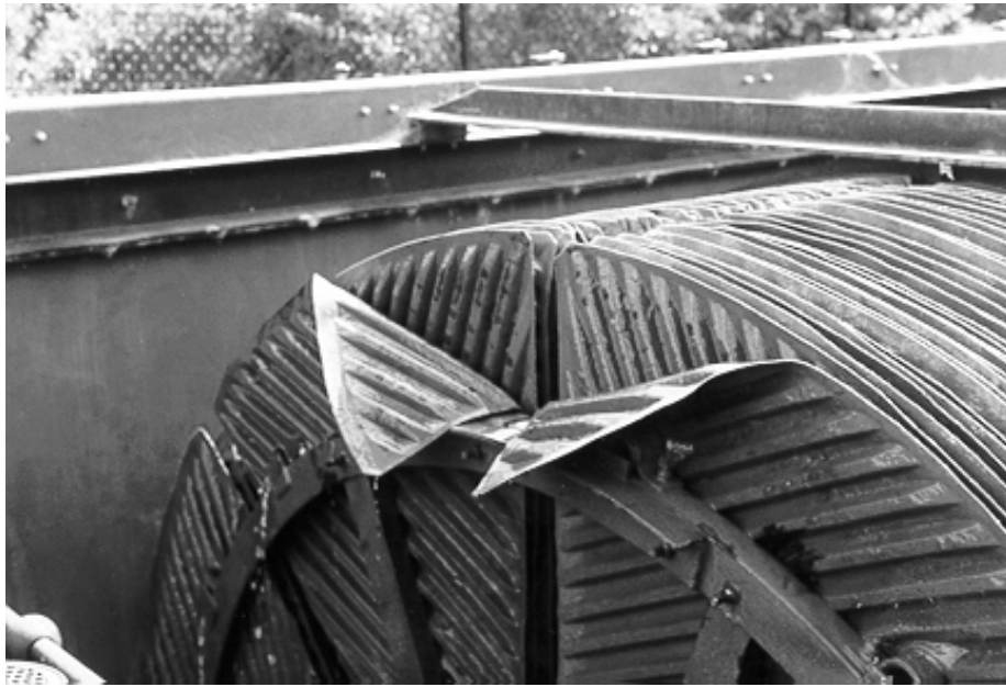
Figure 25 Loss of rigidity on an end media panel
