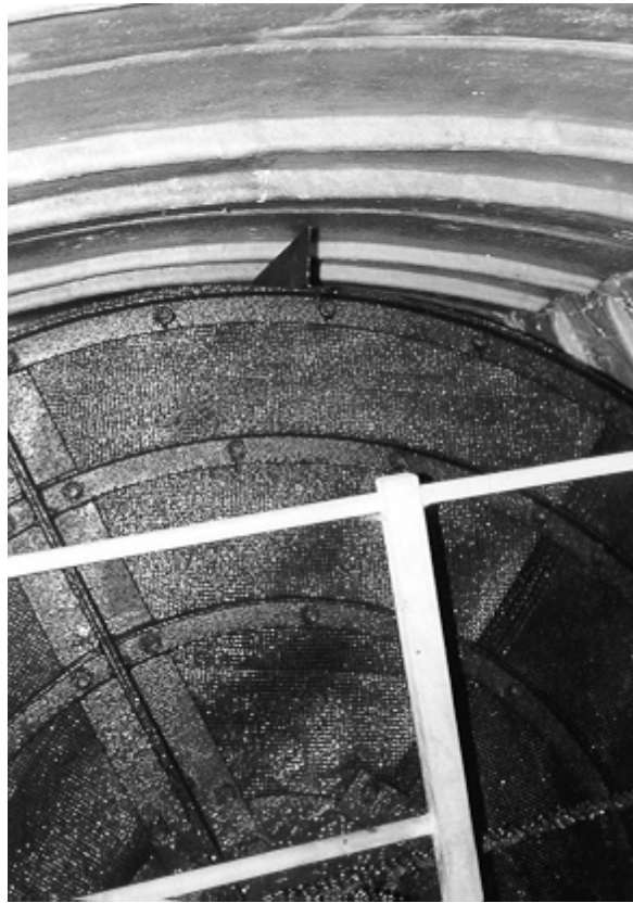
Figure 34 Design arrangement of oldest known operational unit in the UK
