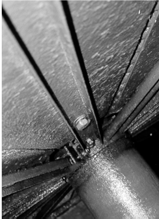
Figure 81 Loose bolt employing spring washer
