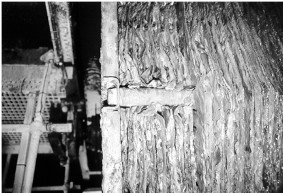
Figure 24 Tearing of High density polypropylene media panels in the vicinity of the support through rod
