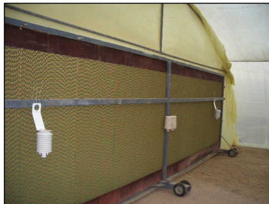
Fig. A1.3: The metallic frame carrying the 2 nd set of evaporative cooling pads
