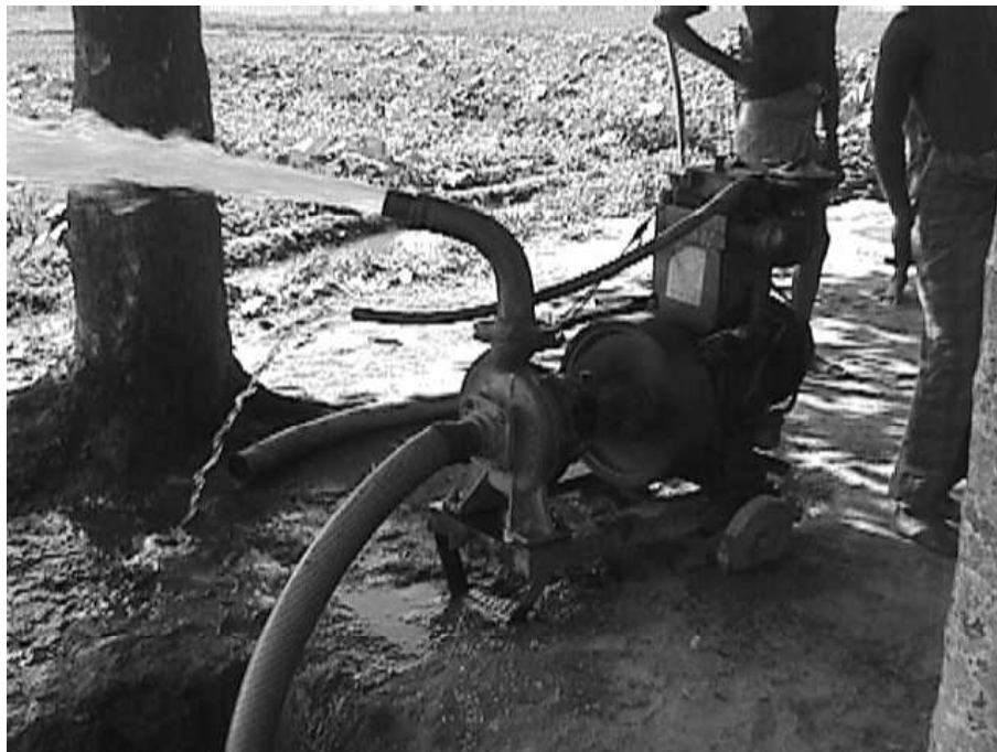
Figure 18: Flow from an Installed 3" Diesel Pump
