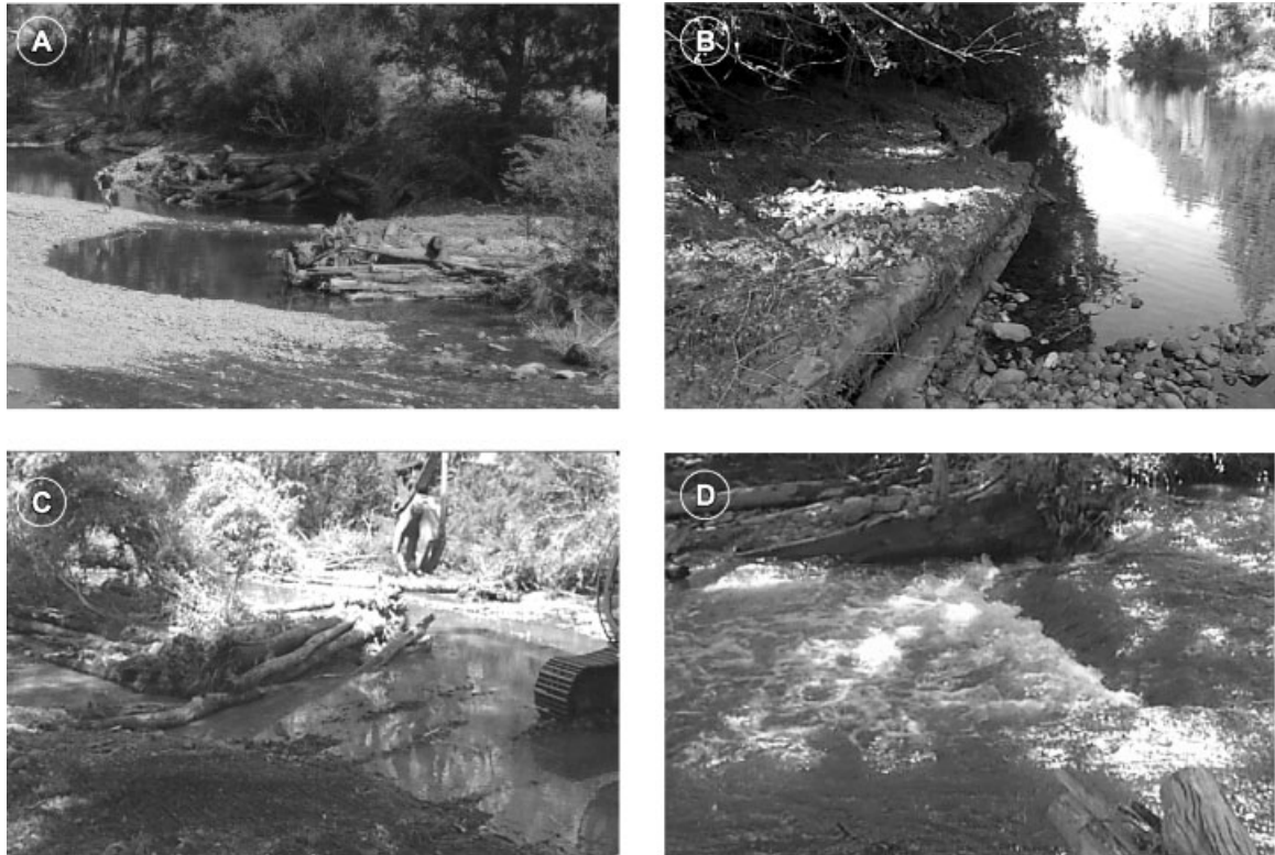
Figure 6. Examples of ELJs constructed in the test reach: (A) deflector jams; (B) bank revetment structure; (C) bar apex jam; (D) log sill bed control spanning between DFJ and BAJ
