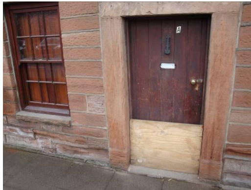
Figure 7 A home-made plywood door-barrier
