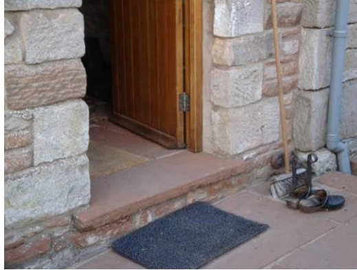
Figure 21 Sandstone walls typical of those found in older buildings in and around Appleby
