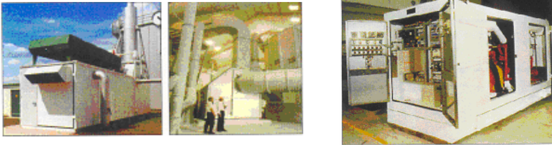
Fig.A.19: Small CHP unit [6]
