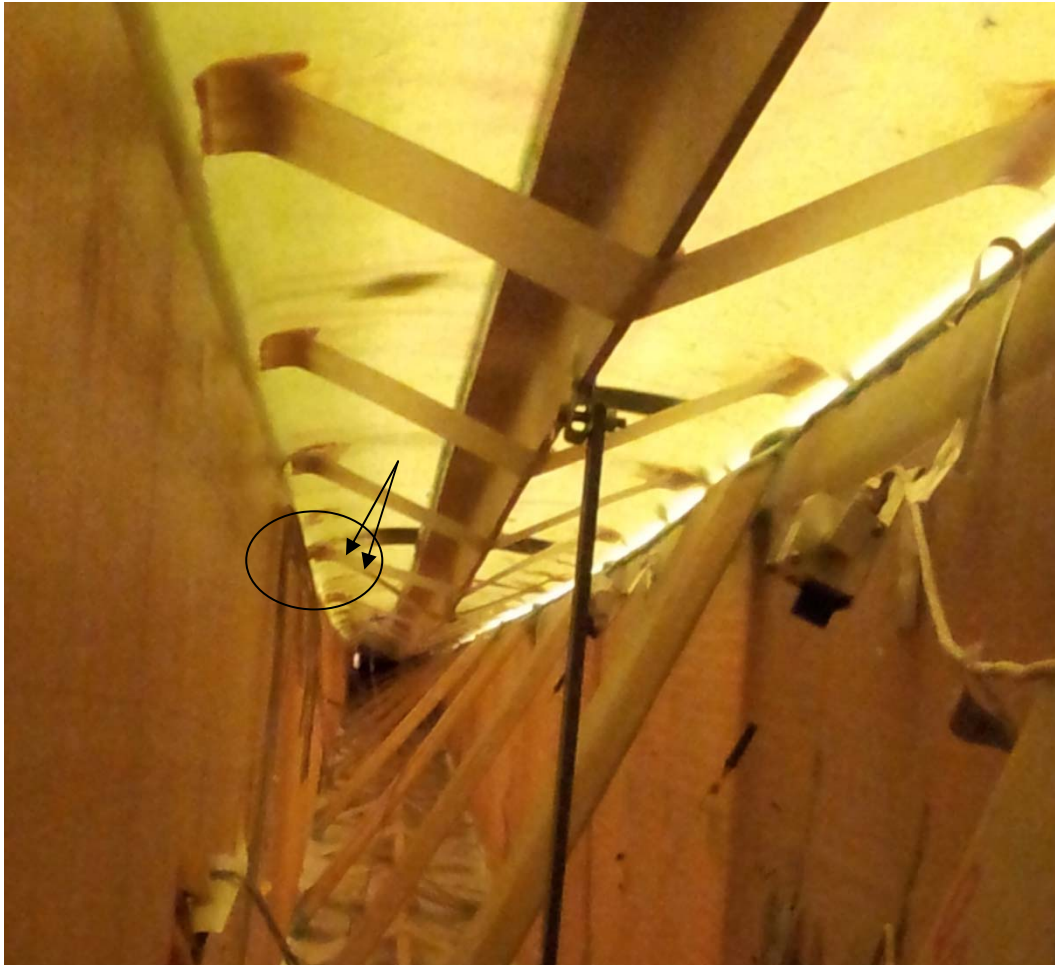
Figure 68 Photo inside the box after the test DMT_2012_05_31_A. the photo is taken inside the box, as it is difficult to get close to where the damage occurred. But examining it closely at the circle, one of the two transverse stiffener has debonded.
