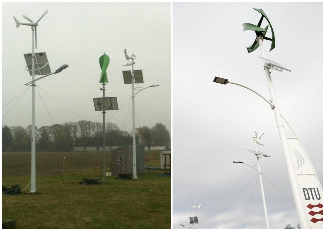
Figure 31 Installed commercial hybrid systems
