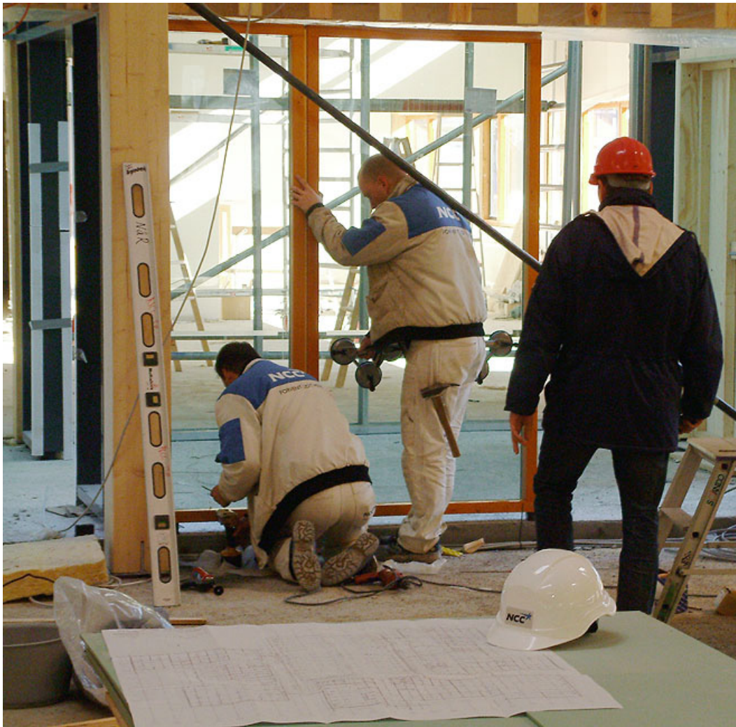
Figure 17: Example of post-modern construction practices
