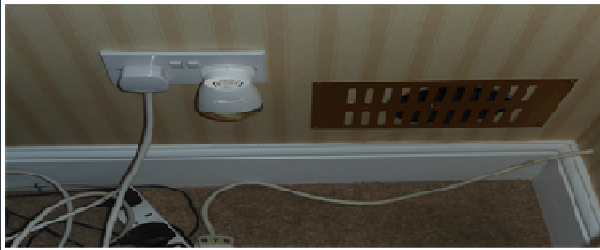
Brian's plug air freshener and safety vent
