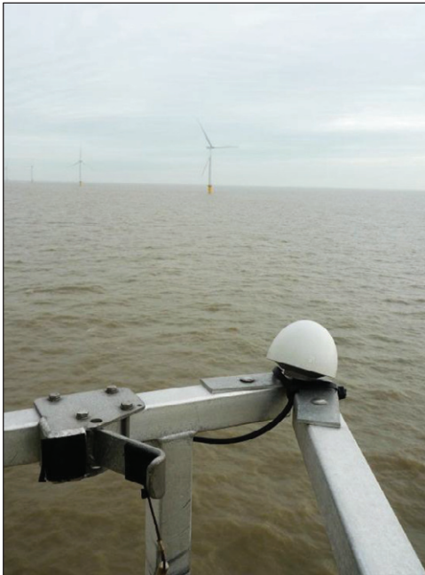
Fig. 3 GPS antenna installed on the service stairs of a wind turbine in Gunfleet Sands.
