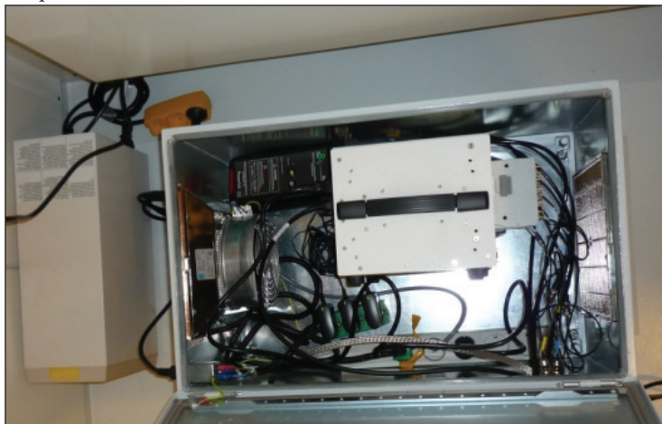
Fig. 6 EMC box installed in the transformer platform at Gunfleet Sands Offshore Wind Farm.
