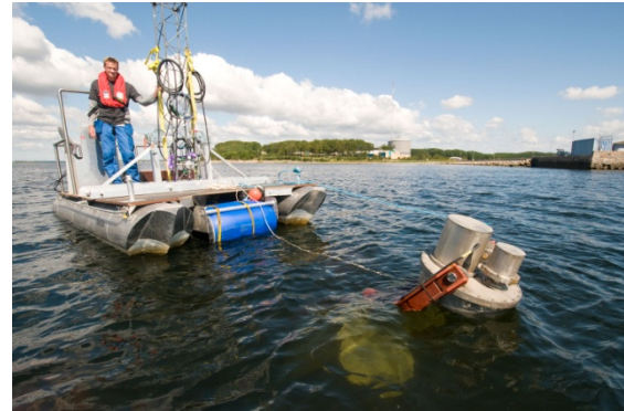
Figure 8 Demonstrator foundation with mast in position 50m from pier, torque arm is lifted with generator box above sea level and sea vessel surrounds mast
