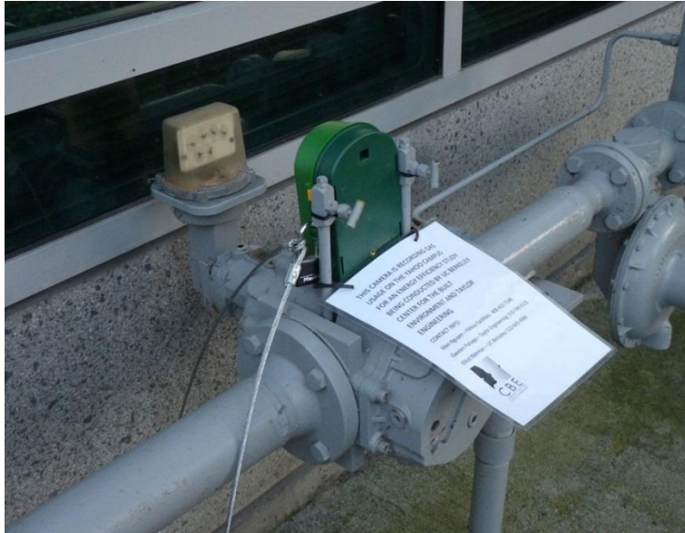
Figure 2.2.5 Gas Meter digital photography
