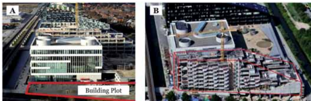
Figure 40: Ørestad Gymnasium before Ørestad School was built. B: Ørestad School under construction.
