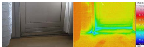
Figure 12: The leaking balcony door in the living room
