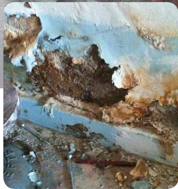
Typical damage due to water penetration through basement walls. Photo: Rimante Andrusiunaite Cox.
