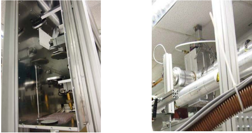
Figure 20. Photographs of the installed receiver box (left) and the RF switch installed in transmission line (right).
