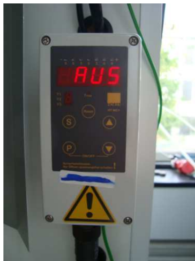
Figure 2.20: Original Control Box for Oven Control
