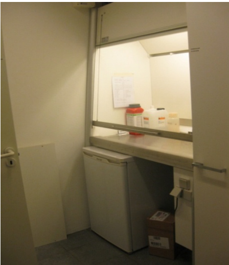
Figure 4.7.2. Fume hood and cupboard for chemicals installed at the laboratory at the research facility.
