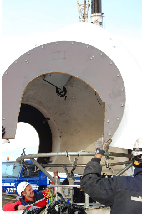
Figure 4.2: Photo of the turbine spinner. The cabinet box is fixed on the inner part of the spinner.
