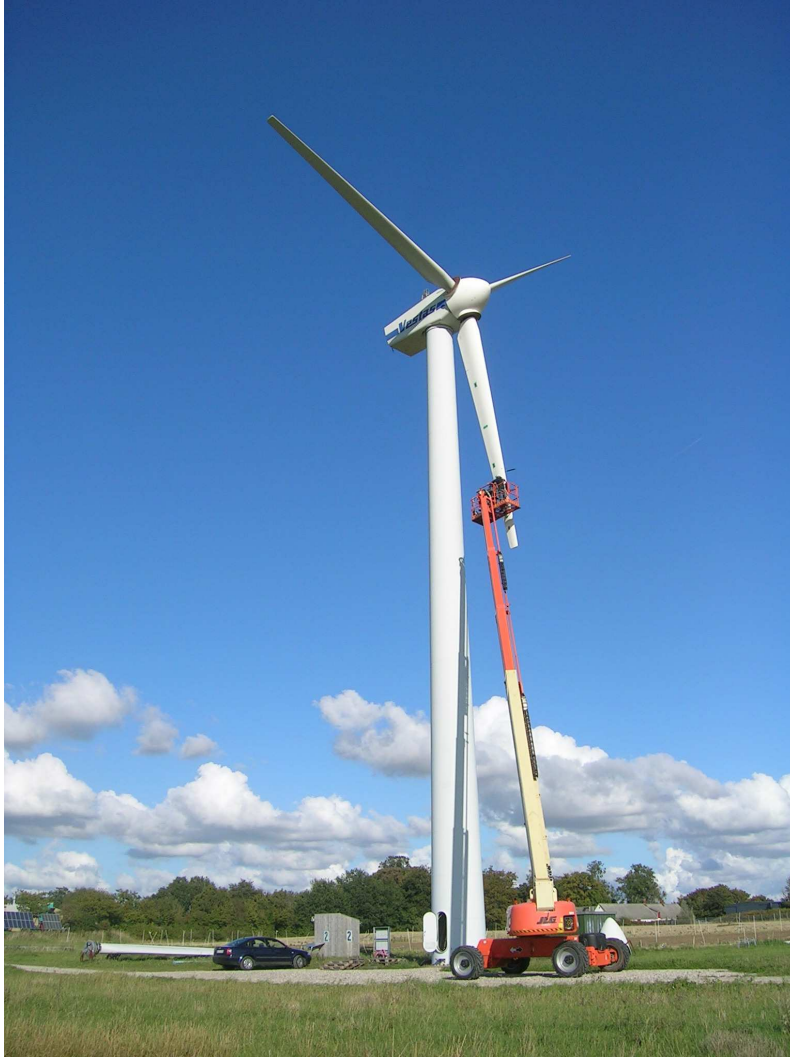
Figure 1.2: Picture of the V27 demonstrator turbine. The cherry picker is used to access the hatches in the blade when servicing the actuators and the sensors.
