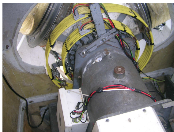
Figure 4.3: Photo of the slip ring which conducts the electricity from the power supplies in the nacelle to the cabinet box in the spinner and the actuators in the blades.
