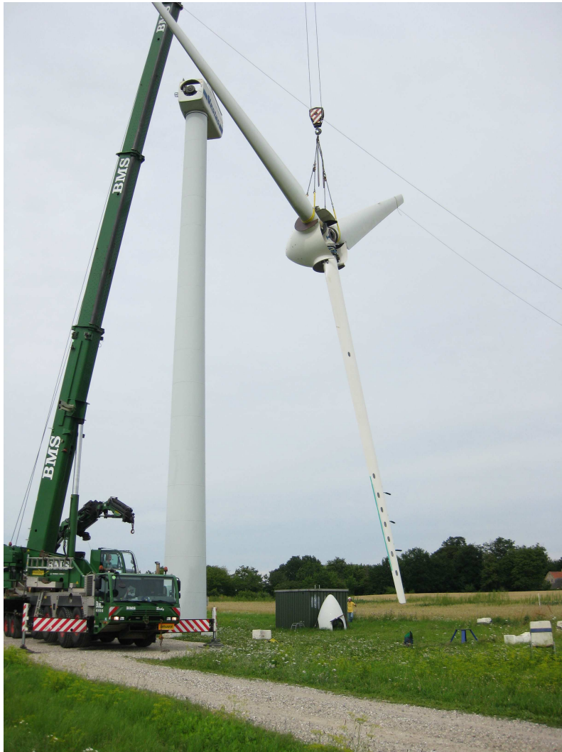
Figure 4.1: Installation of the rotor with the trailing edge flaps on the V27 wind turbine.
