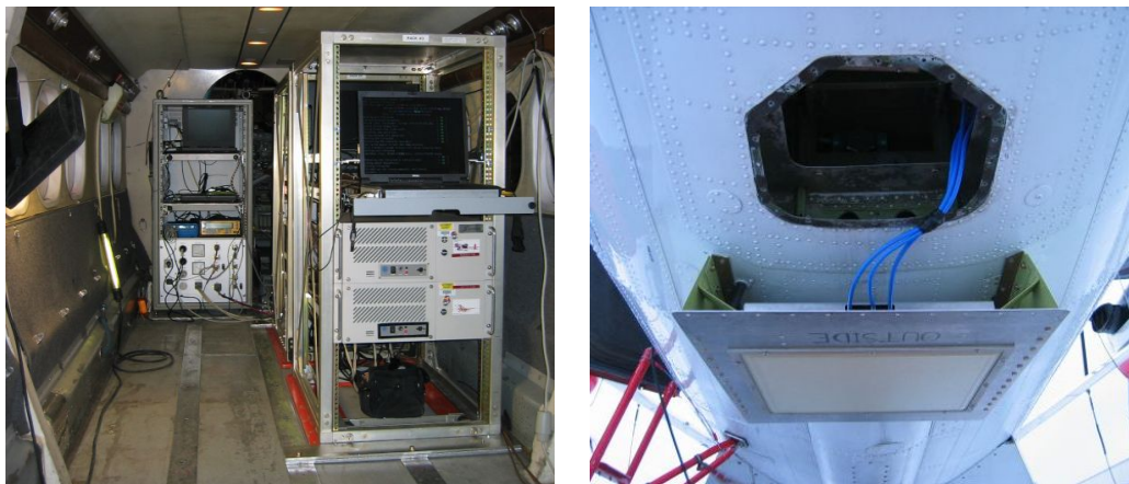
(a) Instrument rack installed in the cabin. D2P to the right and support instrumentation (incl. pc for laser scanner) to the right.
