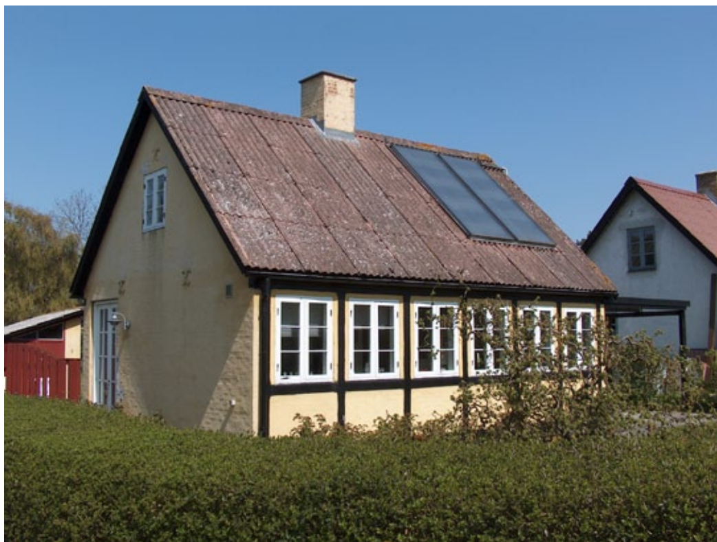
▼ A roof-mounted solar hot water system
