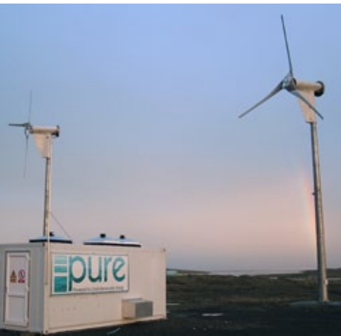
▲ Operational PURE Energy system on Unst, Shetland
