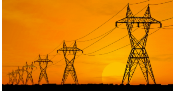
Electricity transmission line.
