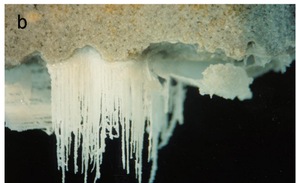
Fig. 3b Calcite needles formed along the crack in the conical outlet space at the bottom of specimen 3-4 with downward flow.
