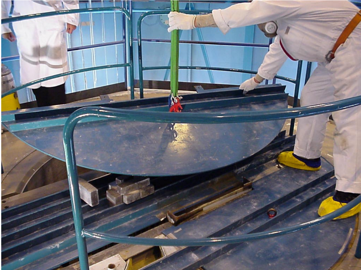
Figure A6. The lifting of the steel lid from the reactor top.
