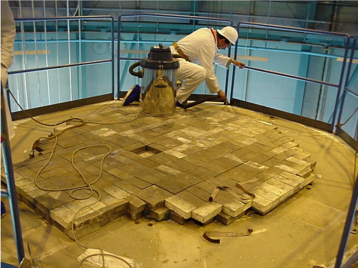
Figure A4. Vacuum cleaning of the lead brick layer below the concrete lid.
