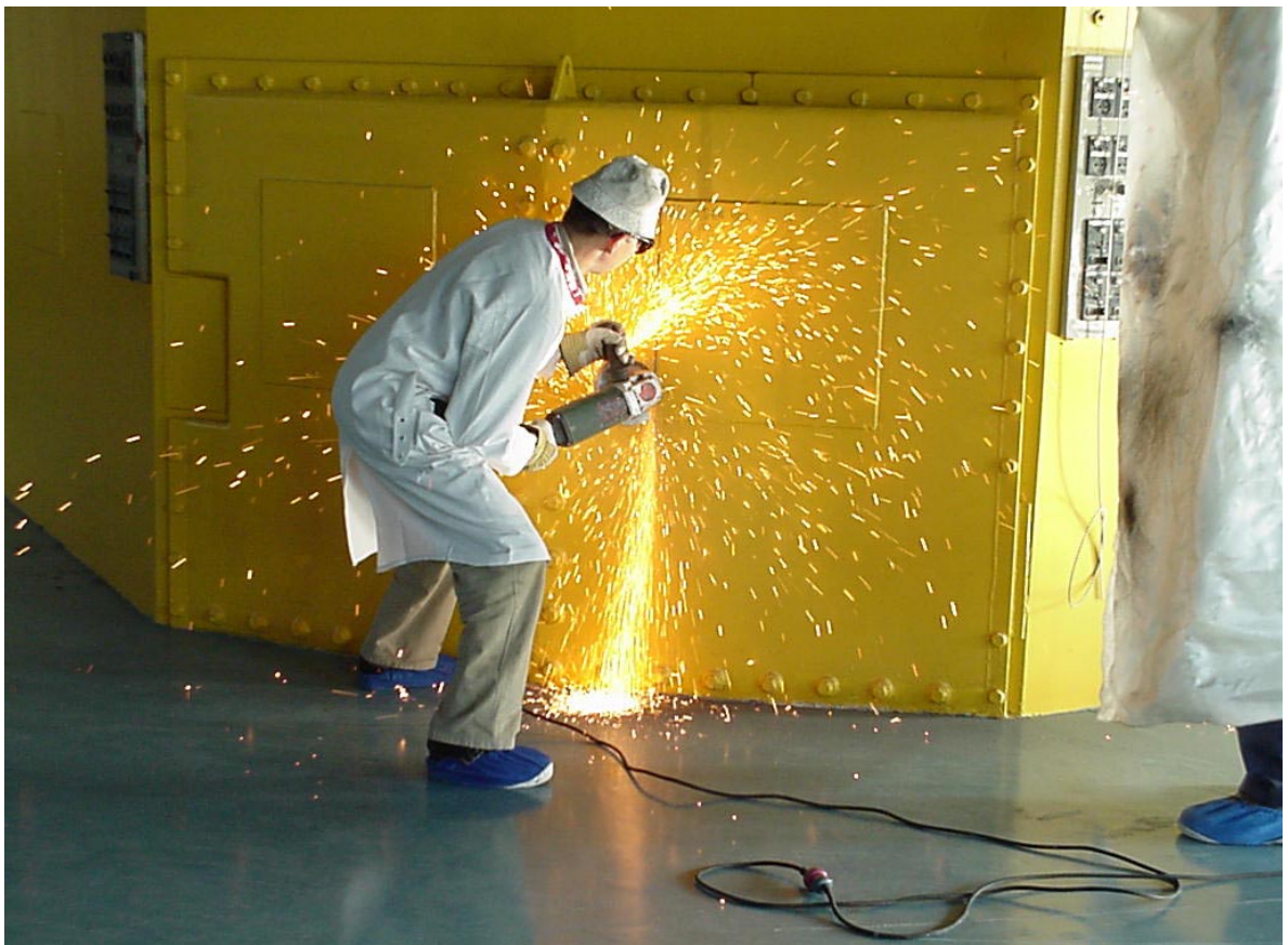
Figure A29. Removal of a steel plate in front of a beam tube.
