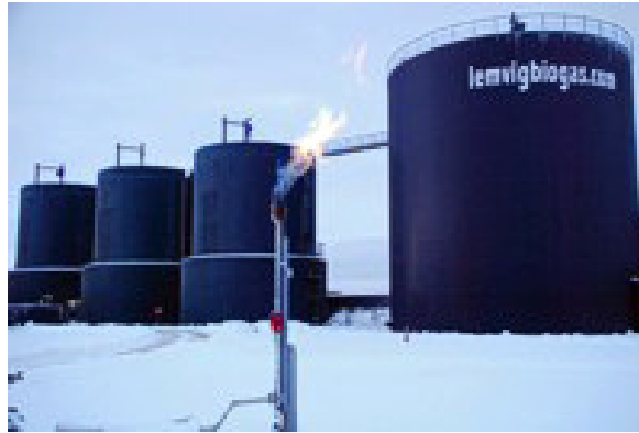
Figure 28. Lemvig biogas plant (17,500 m 3 reactor volume)
