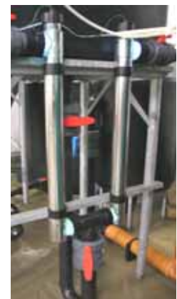
Fig. 2.3. UV treatment system 2005-2007
