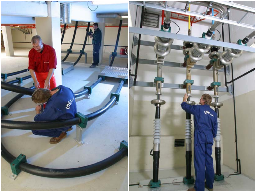
Figure 6. The HTS power cable installed in the basement of the Amager substation and view of the cable termination
