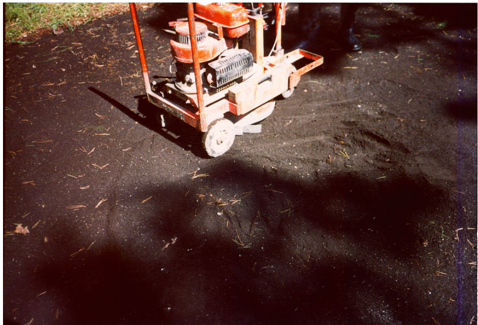
Plate 5.2. The asphalt scraper working on the contaminated pavement. As can be faintly seen from the picture, the road is covered with a powder of loosened asphalt particles after the operation.
