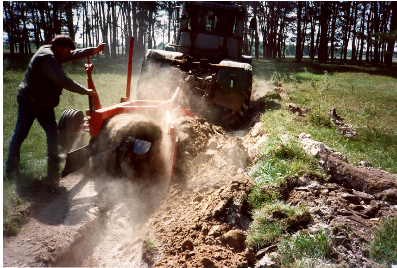
Plate 4.1. The plough in use in the Novo Bobovic area. The skim furrow is made on the left by the skim coultter while the main coultter simultaneously creates the deeper trench in which the top layer is buried. The plough is here going too deep and the person behind it is trying to adjust the ploughing depth.
