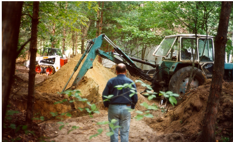
Plate 3.3. Excavator digging holes for waste burial in the forest. The sand is placed in a pile on the cleaned ground and the topsoil lies ready on the other side of the hole.
