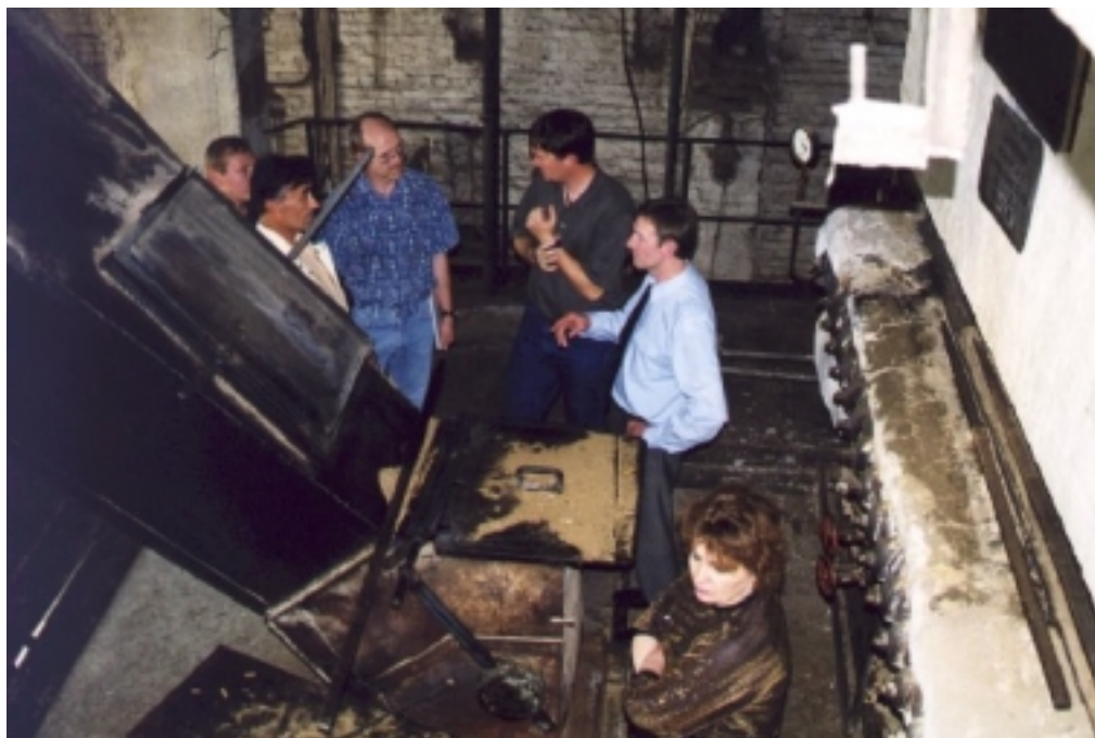
Figure 1.3 The photo shows the chute where the fuel is stored right before feeding into the boiler.
