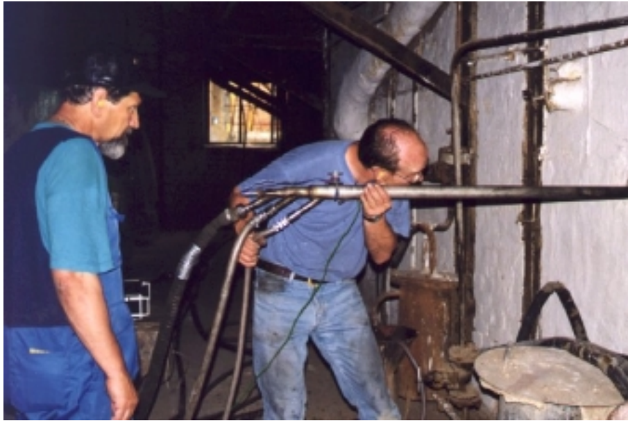
Figure 2.1 Measurement of the combustion temperature in the boiler using a suction pyrometer.
