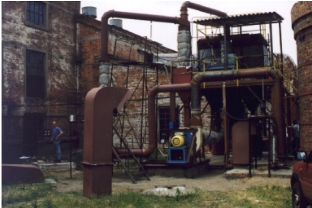
Figure 1.4 Baghouse built over the underground flue gas duct. The boiler building to the left and the stack to the right.
