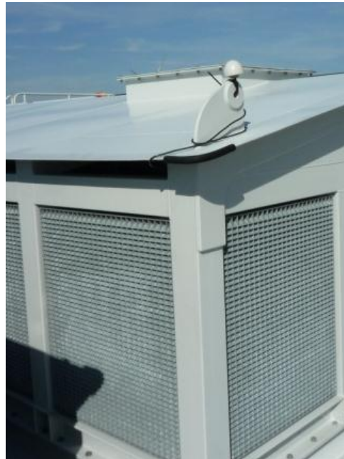
Fig. 4 GPS antenna installed on the platform upper level in Gunfleet Sands.
