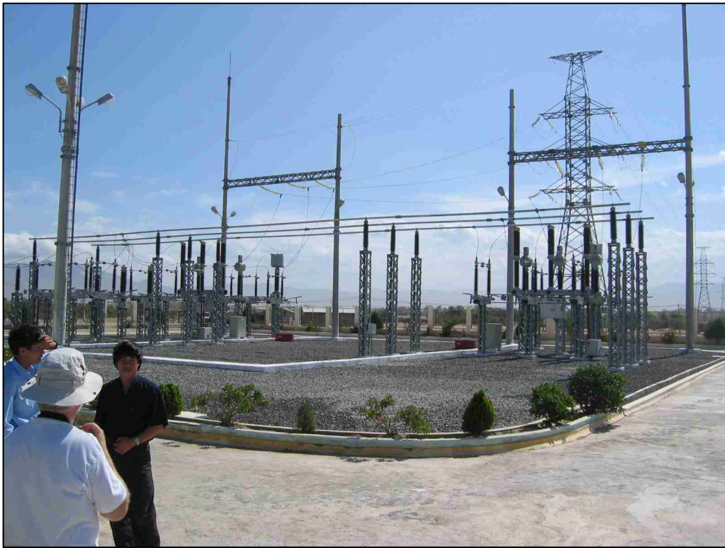
Figure 9: The power sub-station at the Phouc Minh site. (Photo: RISO)
