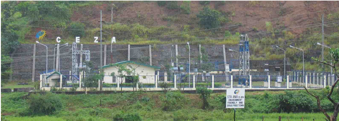
Figure 5 CEZA sub-station feeding the town of Sta Ana
