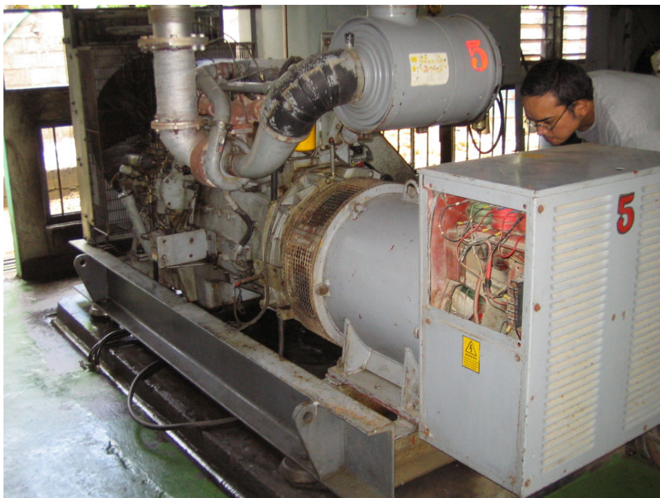
Figure 15 Dale-Perkins diesel generator in Dinagat power plant
