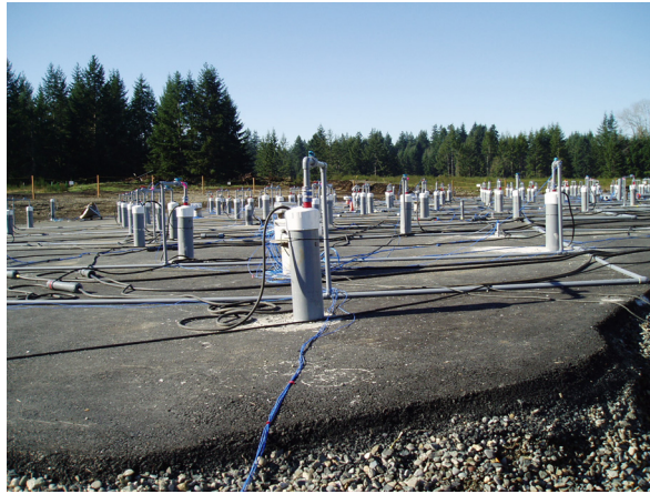
Figure 8. Electrical resistance heating (ERH) at Ft. Lewis EGDY, 2005. Electrodes inserted at a distance of approximately 5 m.
