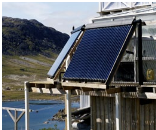
Solar Hot Water Panels, Qaqortoq, Greenland 13
