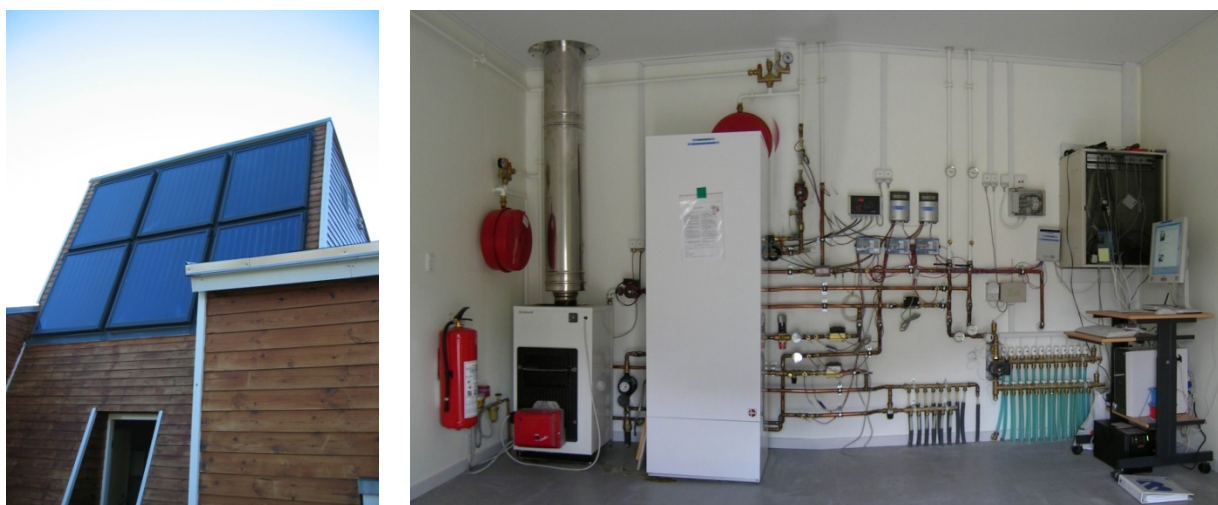
Figure 5.3. Flat-plate solar collectors on the Low Energy House and the installations in the boiler room.
