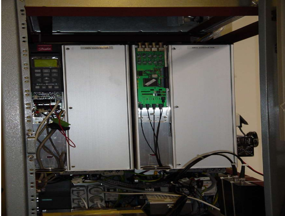
Figure 36 Prototype rack with power converters, controller and interfacing equipment (power converters are shown)
