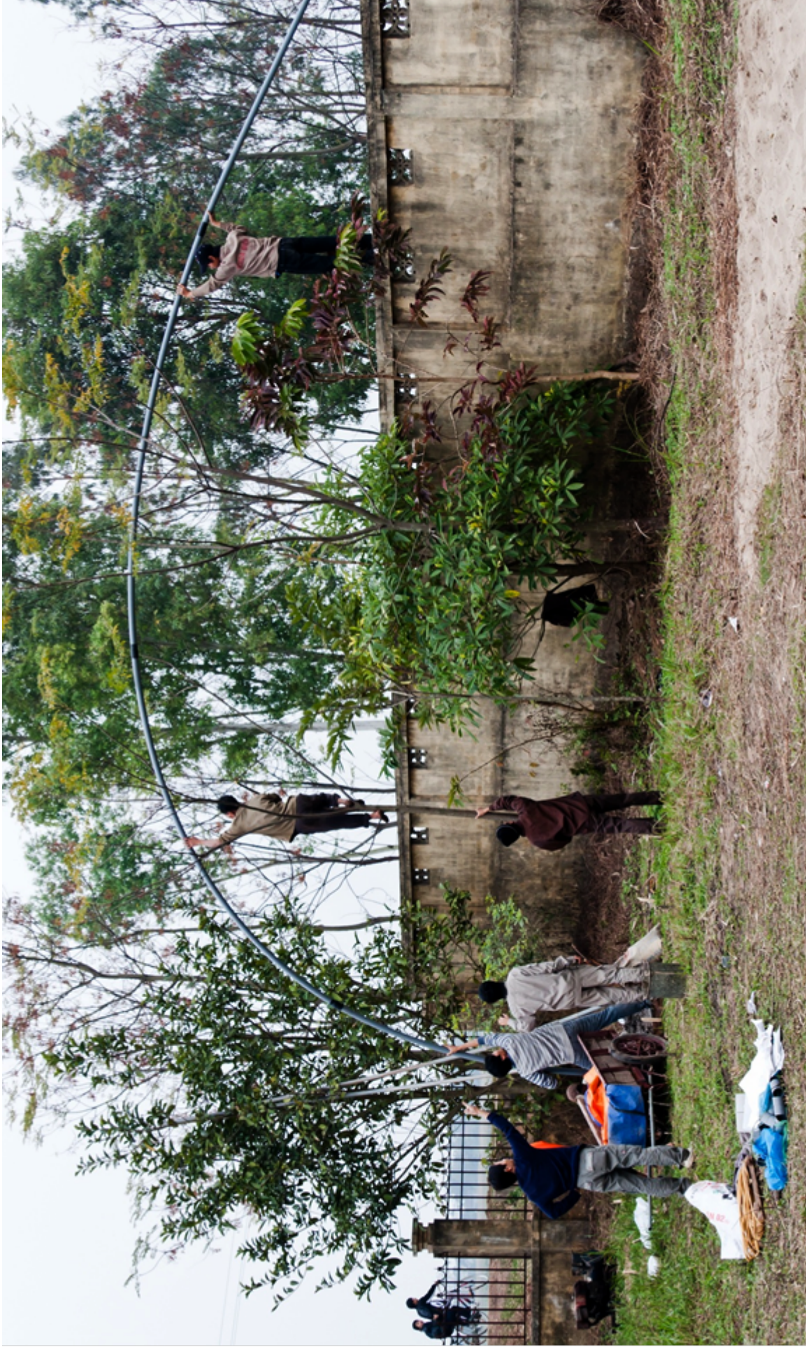
Installation of well screen at the Van Coc site of the School Transect of the VietAS project. After the borehole has been made by water jetting, the hole is open for a very short time due to a very thin mud cake formed by the natural clay content of the Red River sediments. Because the time is so short, the entire screen and casing is assembled into one long string, which is then rapidly inserted immediately after the water jetting equipment has been retracted. Critical as it is – everyone around participates on the ground, in the trees and on the wall. Wells down to >40 meters can be screened and cased in this fashion.
