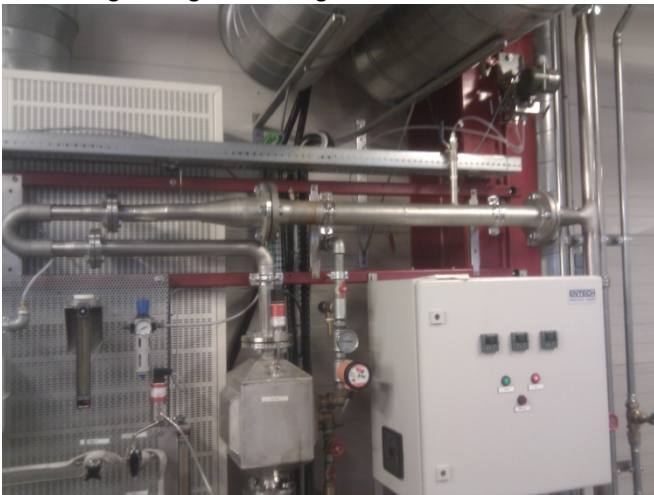
Figure 39 The heat exchanger HE2 is seen at the bottom center. Downstream of HE2 the horizontal piping contains the venturi meter U1.
