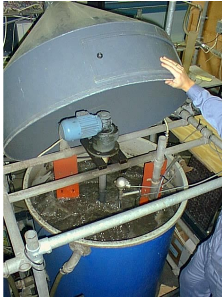
Aerated Tank No.2
