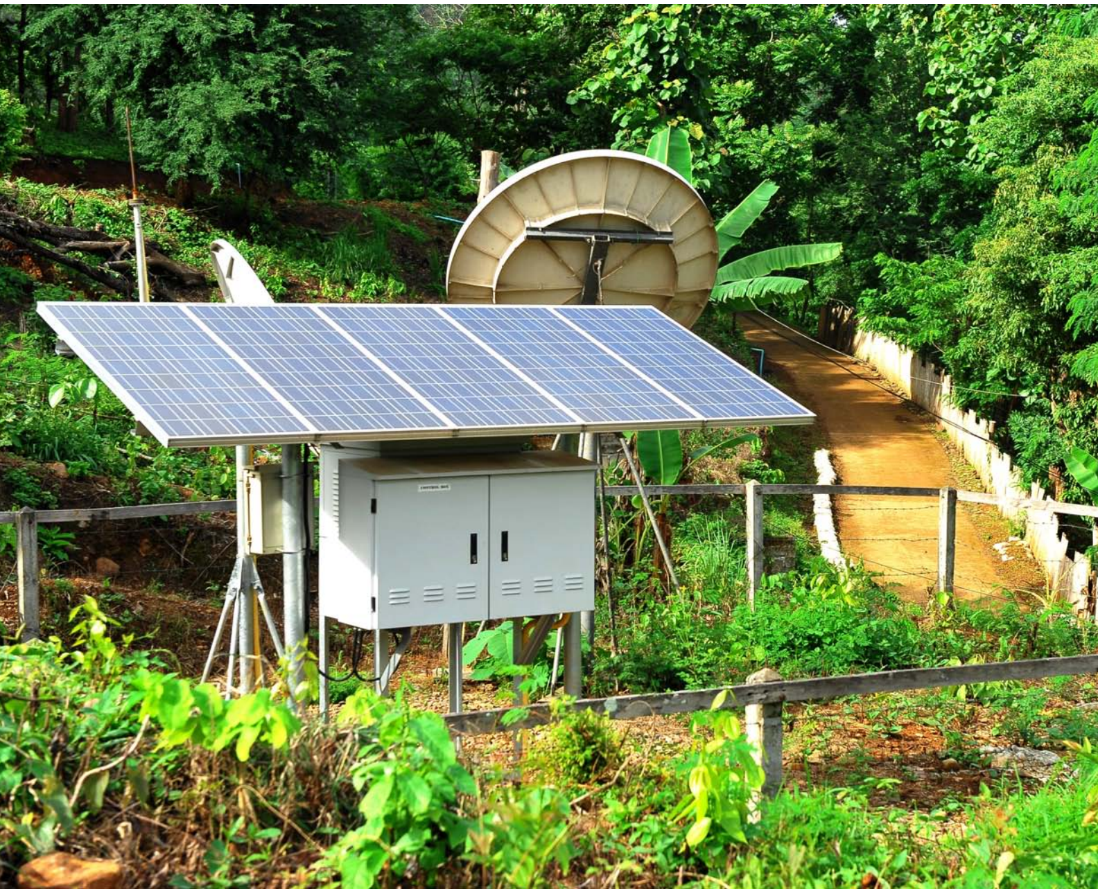
Solar PV used to power village communications Photo: UNEP internal archive
