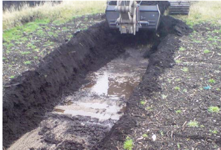
Figure 3.2. Excavation of window 1.2. Water in the gas distribution layer is clearly visible.
