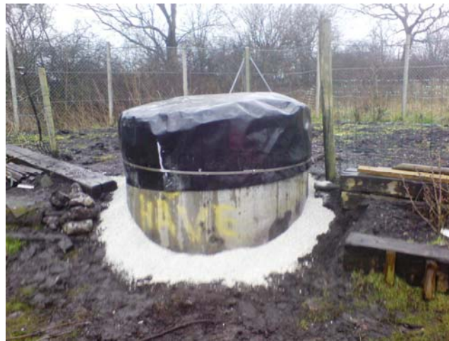
Figure 3.1. Leachate well with edge sealed with bentonite.
