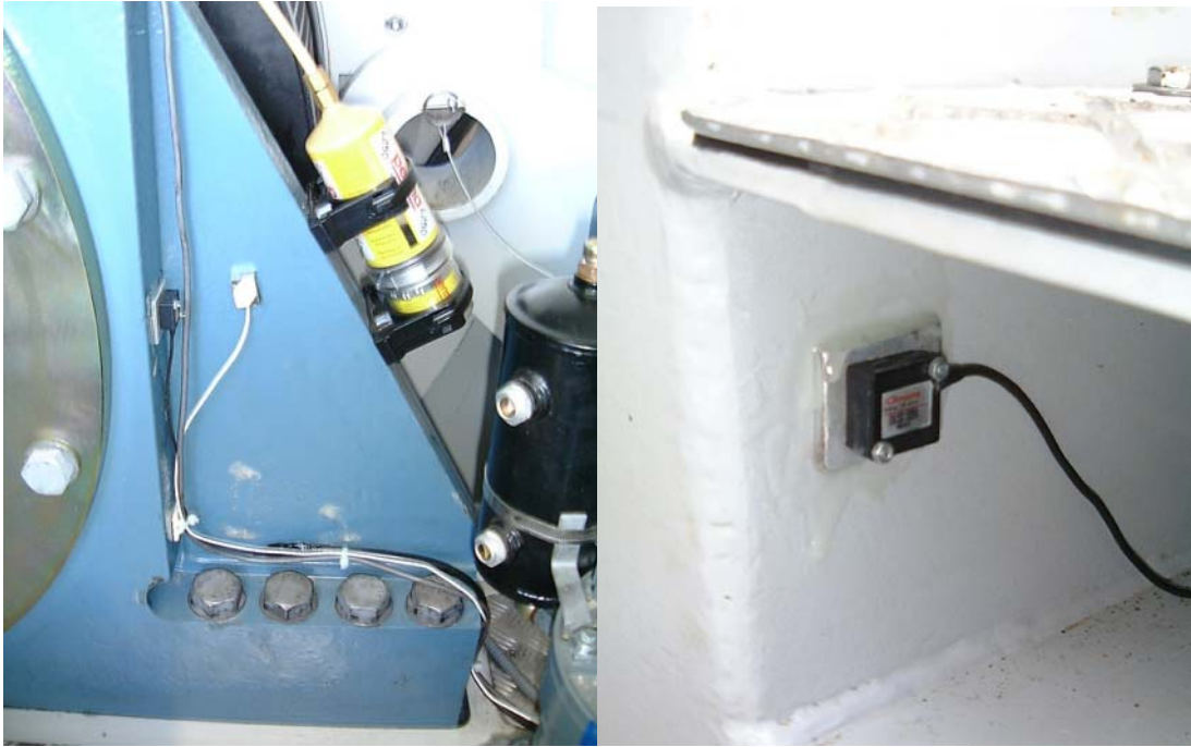
Figure 5: Acceleration sensors on the supporting structure of Turbine 7.
