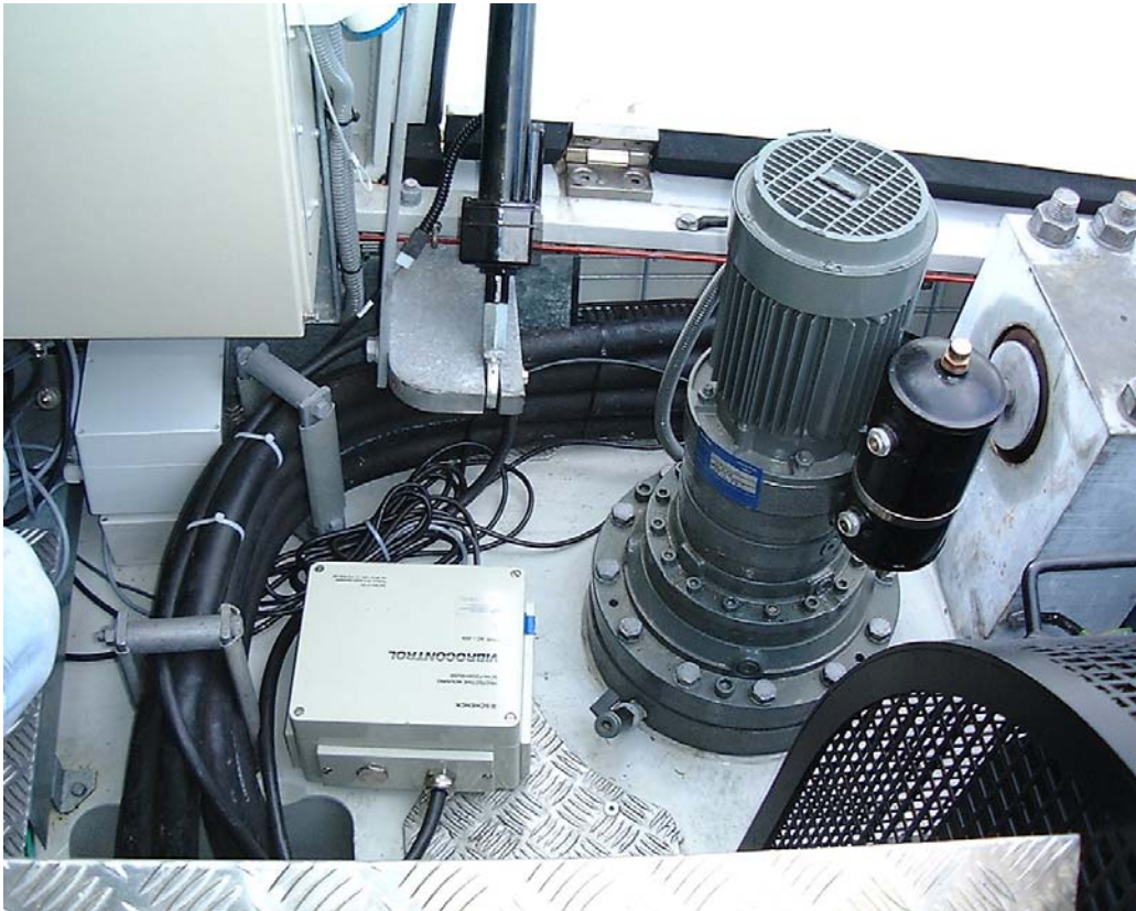
Figure 8: Connection box in the nacelle of Turbine 7.
