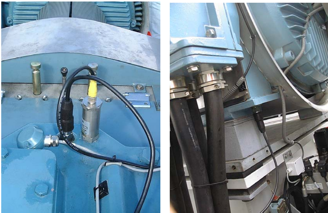
Figure 6: Vibration sensors on Gearbox and Generator
