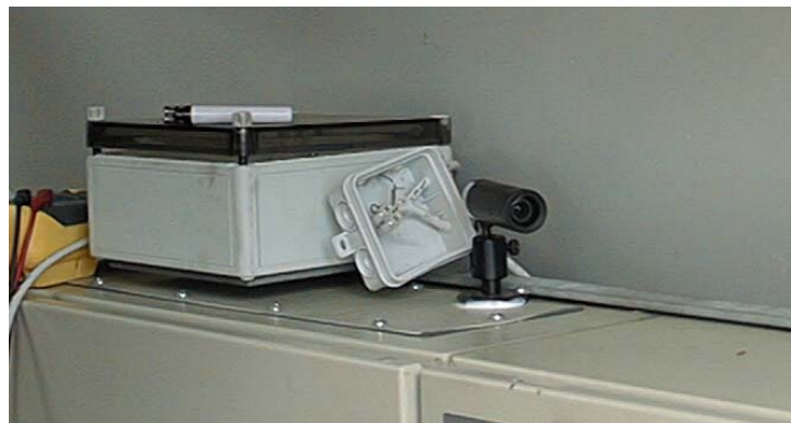
Figure 31: The inside webcam to monitor the nacelle of turbine 7.
