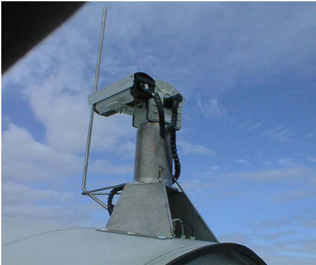
Figure 30: The Overspeed video camera, with full pan-tilt-zoom functionality. The long metal rod on the side is the lightning protection for the camera.
