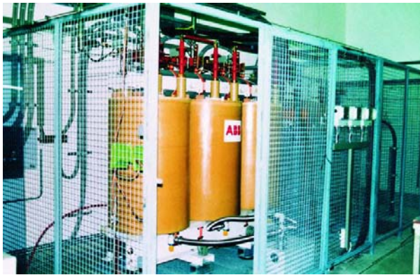
Figure 1. A 1 MW HTS transformer tested in the public network (courtesy of American Superconductor Corp.)
