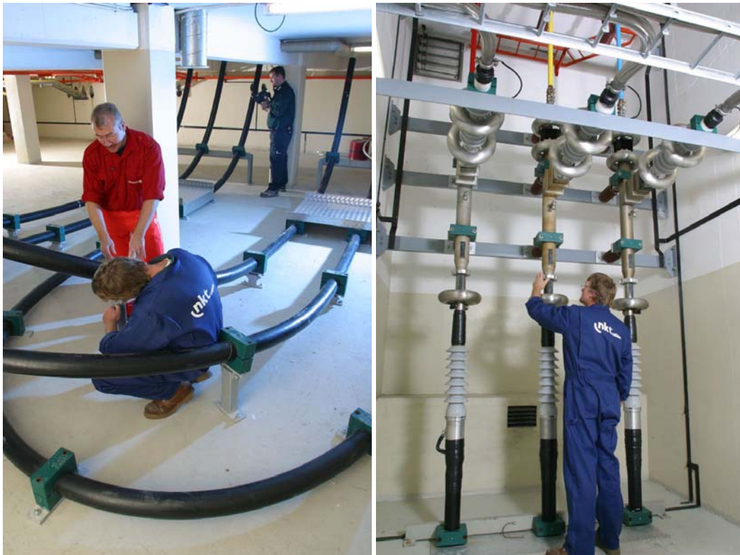
Figure 6. The HTS power cable installed in the basement of the Amager substation and view of the cable termination
