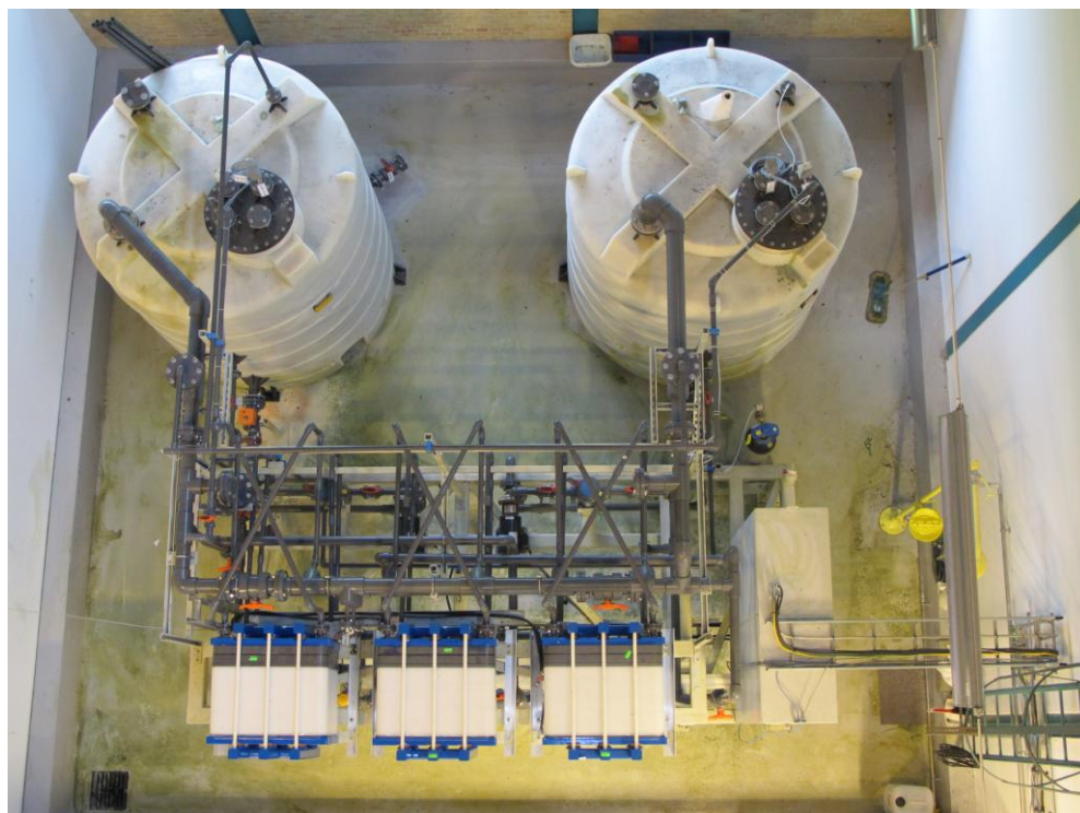
Figure 4 Vanadium battery installation seen from above: electrolyte tanks in the back, 3 cell stacks at the front.
