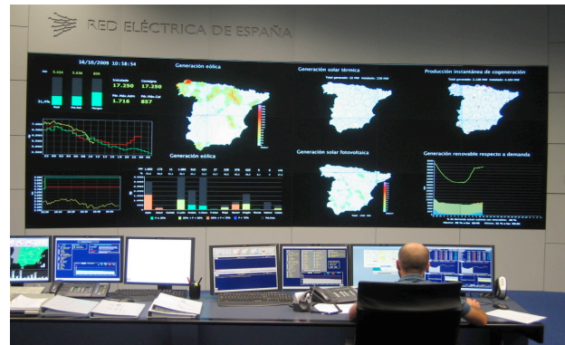
Figure 9: Control Centre for Renewable Energies of Spain (CECRE).
